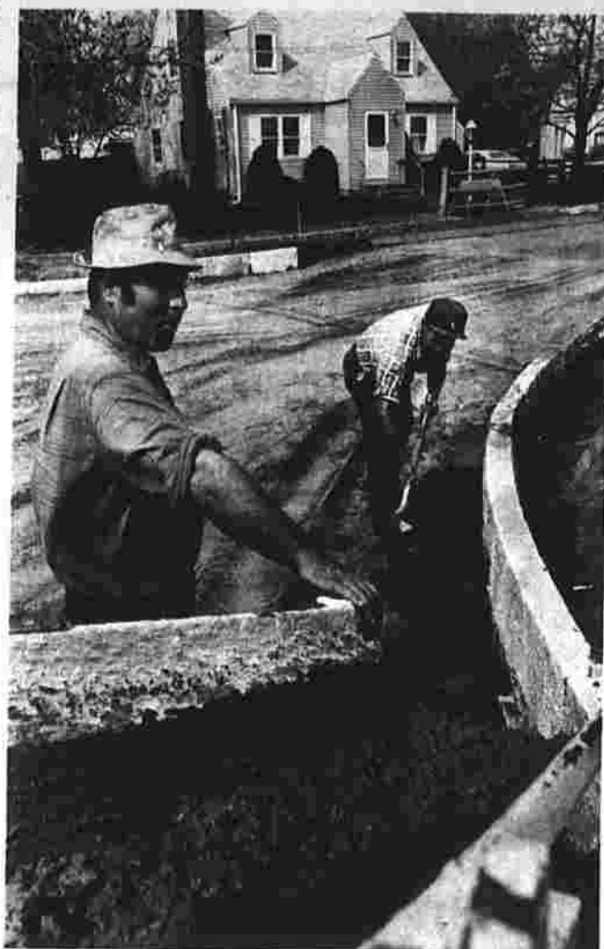
Dominic Zaino, left, and Joseph Pullo, employees of Corsetti Construction Inc., pour cement to anchor new curbs that will be installed on Adams St. The work is part of the Urban Systems Project to upgrade both Adams St. and W. Middle Tpk. (Herald photo by Dunn)
